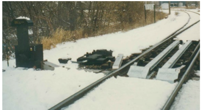
Forced hot air directed through ductwork melts snow and ice from switch components.
