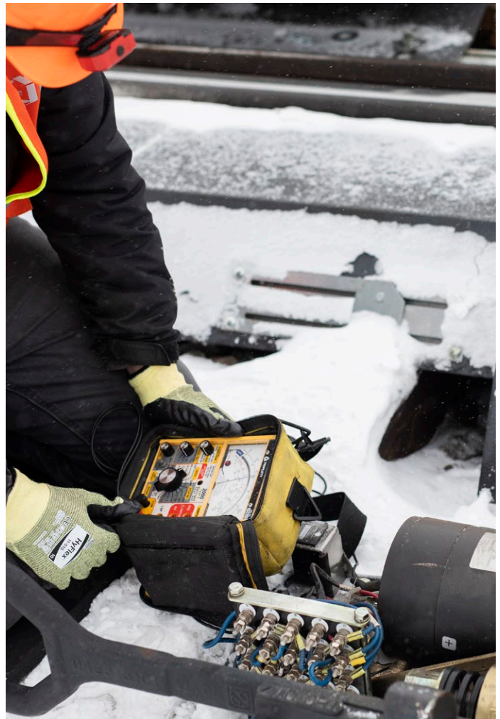
CPKC's Stephen, Alta. weather station includes a remote viewing camera to monitor surrounding snow conditions. The weather station provides real-time data that measures the atmospheric conditions CPKC trains will encounter in the area.
